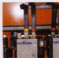
Electrical: Termination problem on yellow phase
